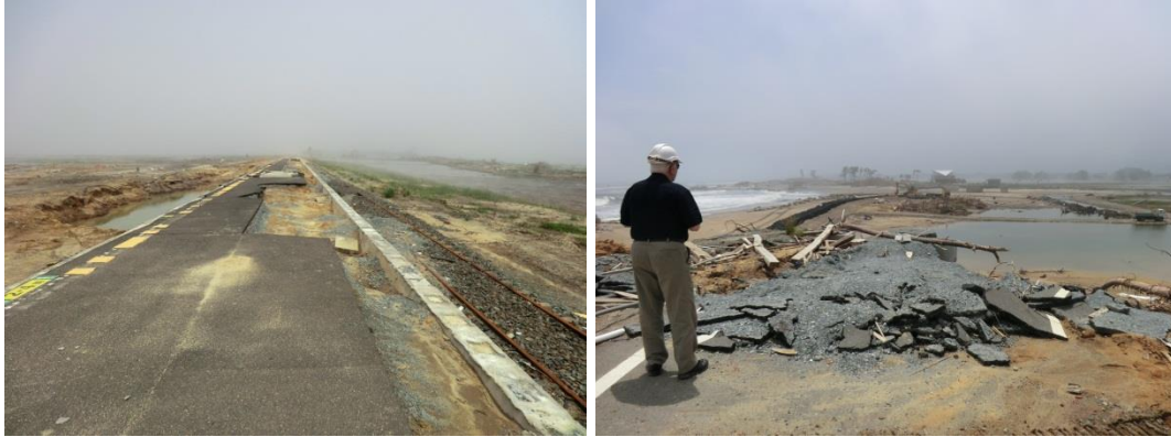
Figure 5. Left: railroad bed and rail on either side of a commuter rail platform were scoured away in the Tohoku earthquake. Right: 1 mile of Japan coastal Route 38 had bridges and roadway on levees destroyed by the 2011 Tohoku tsunami.
